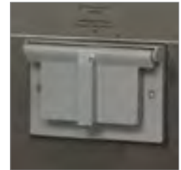
Duplex and/or GFI Outlets
